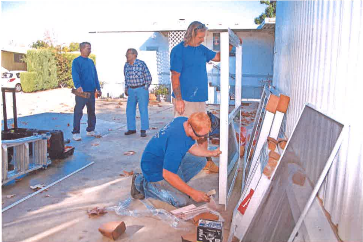
From left: Tom Duffey, owner of Duffey's Mobile Home Service, talks with Henry "Hank" Heeber as Jim Mitchell and Shawn Speer get ready to install a new window on his Thousand Oaks mobile home. JOE LUMAYA/SPECIAL TO THE STAR
